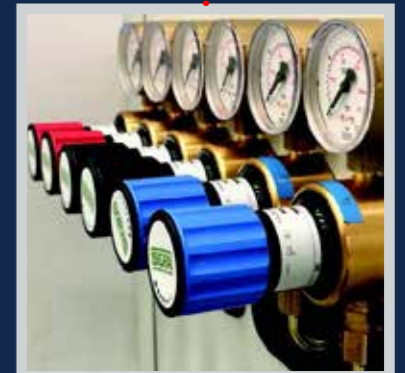
Pannello controllo gas Gas distribution manifold
