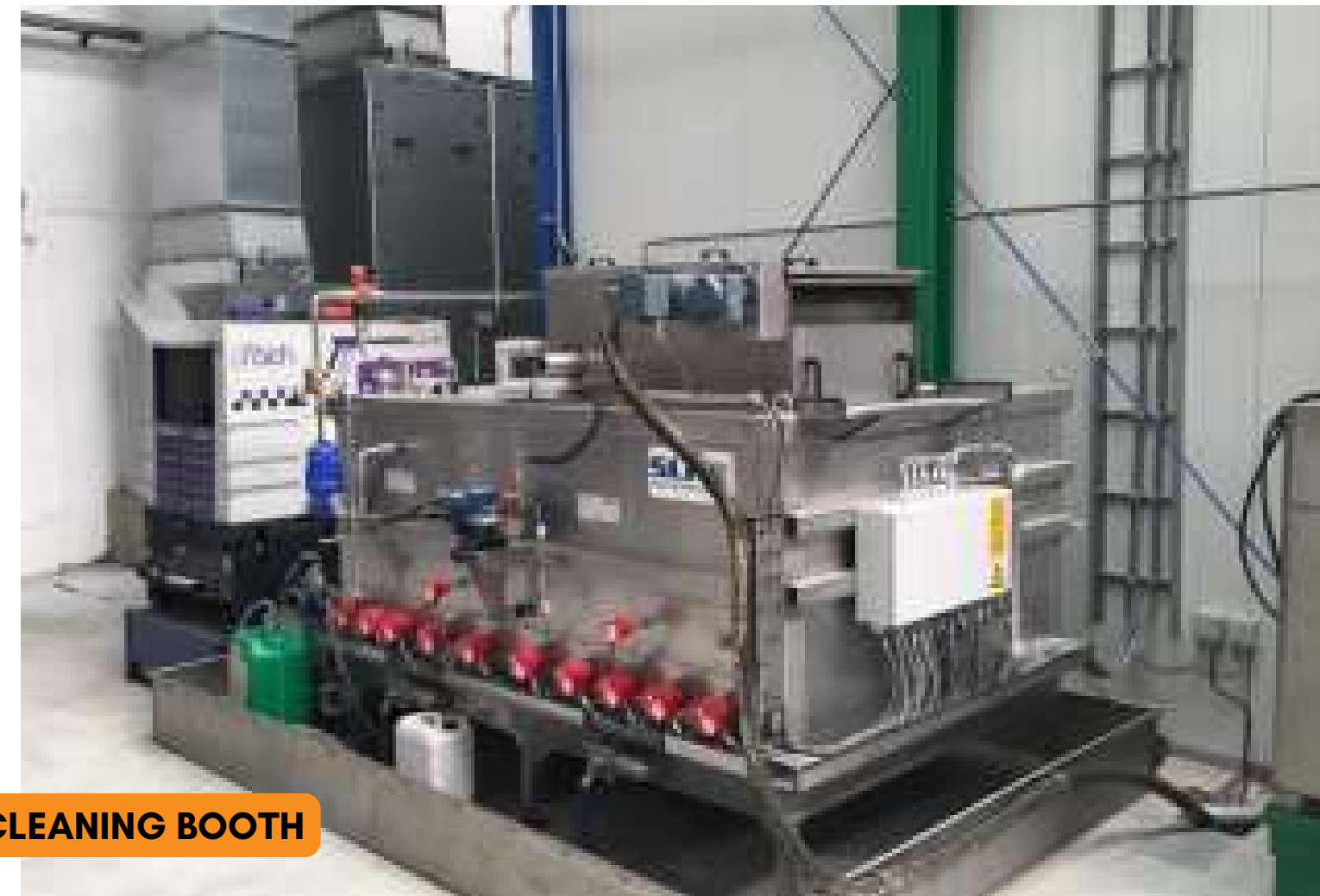
Process water treatment system
