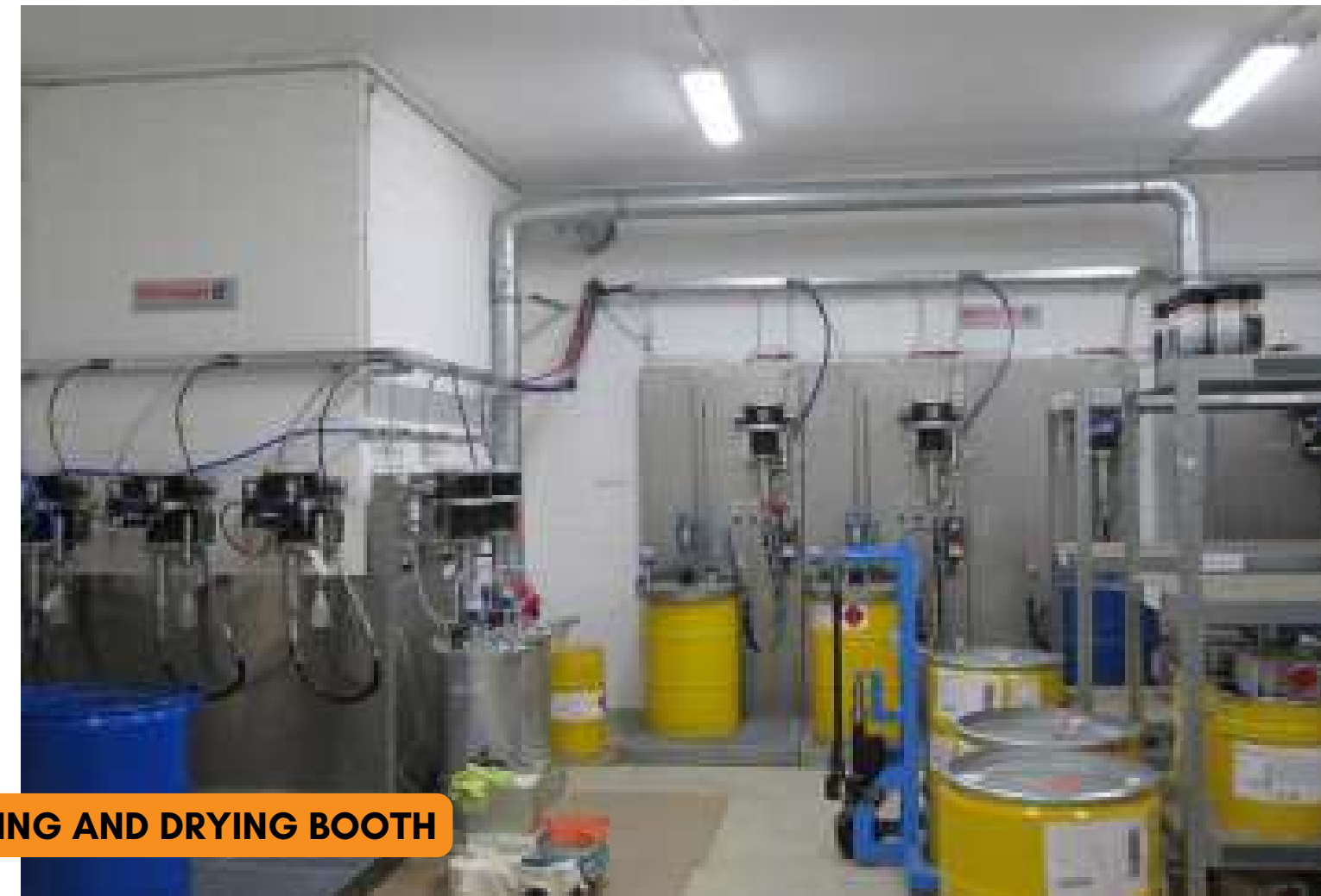
Adjacent paint storage room to store flammable liquids (solvent-based paints)
