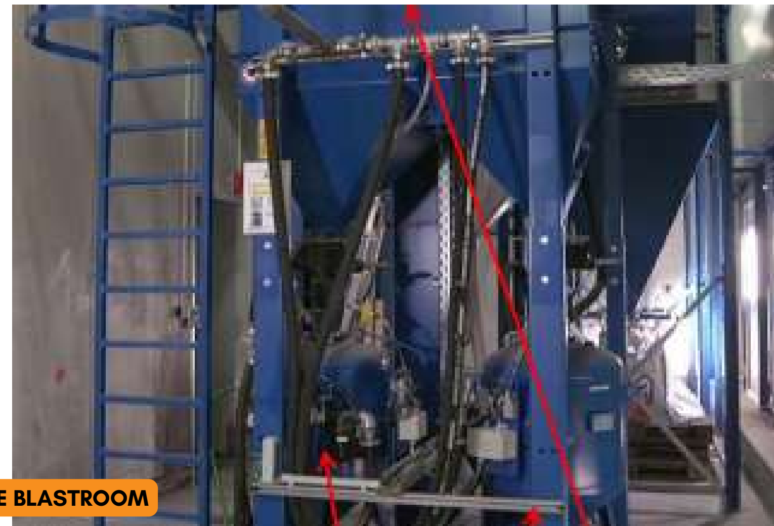
Two pressure blast pots / Media silo
