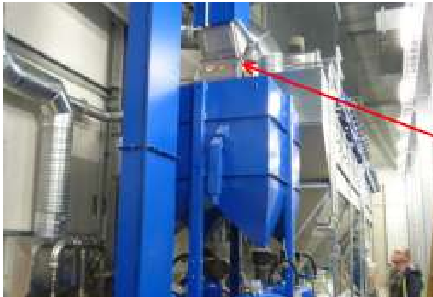
Machine room with filter unit
