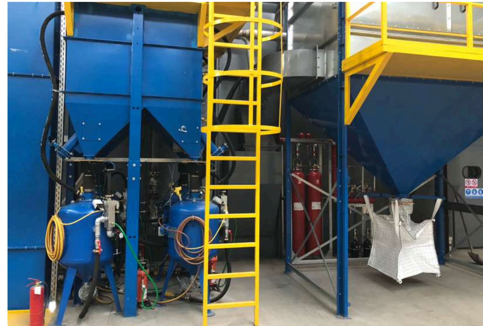
Abrasive silo with four pressure sandblasters
