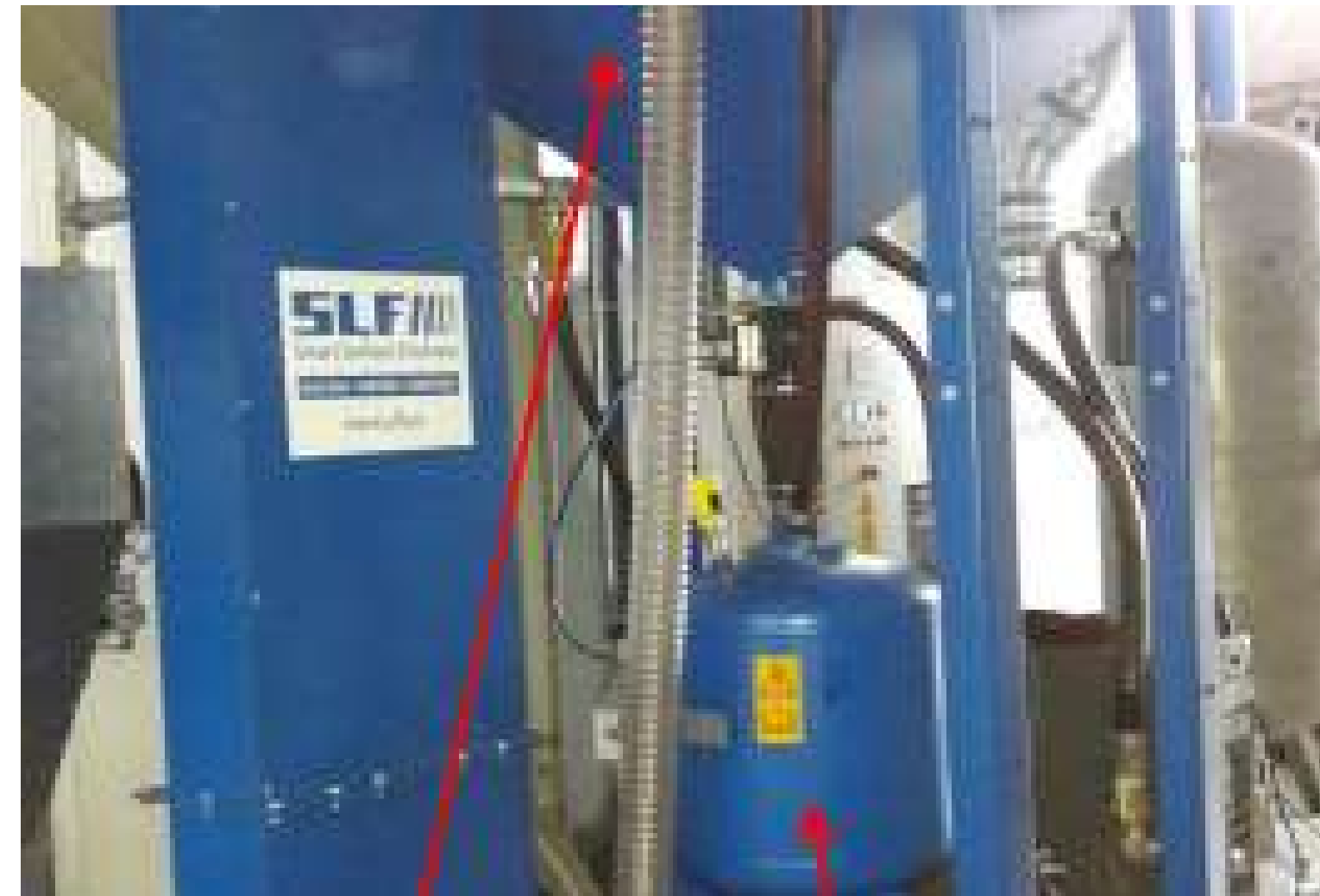
Media silo and pressure blast pot
