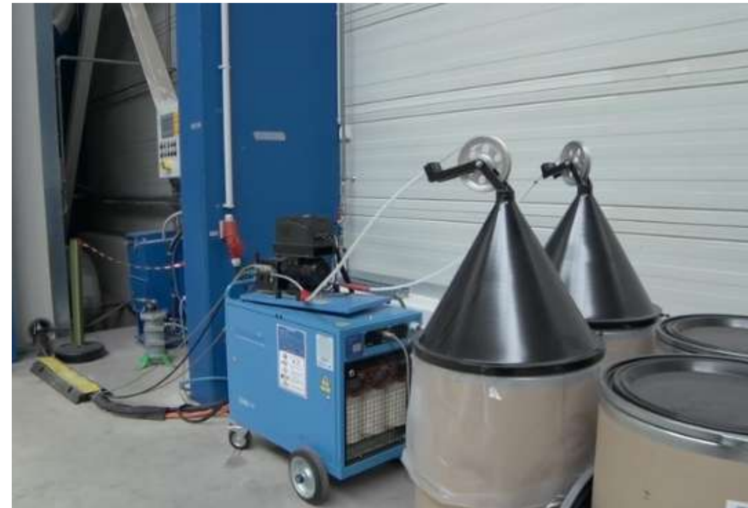
Zinc fill station
