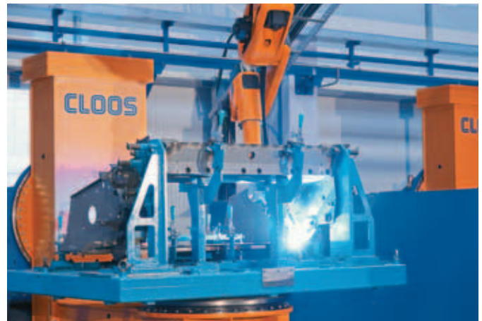
Optimum accessibility of the component by exact positioning of component and robots
